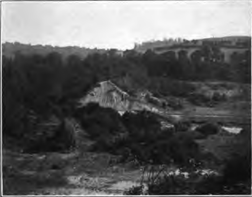
A. SOUTH FORK AND WASHED AWAY DAM.
